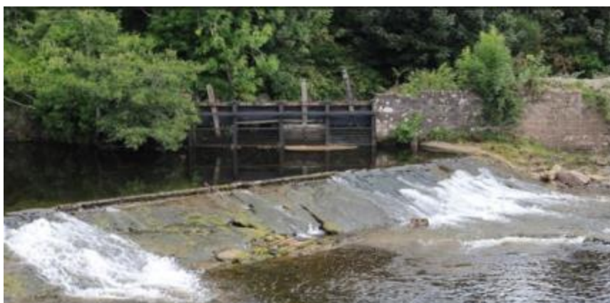
Figure 7 – The river at diminished flows showing the gates and minimal flow immediately downstream of the gates
